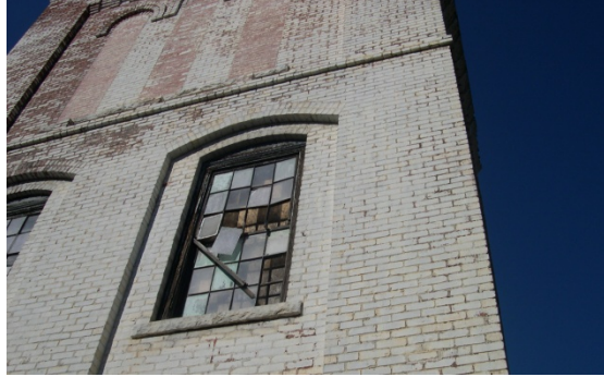
Image 3.6: View of the window that needs to be replaced
