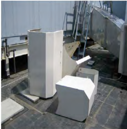
Figure 7: Original Fan Covers – “Totally Enclosed-Fan Cooled”
